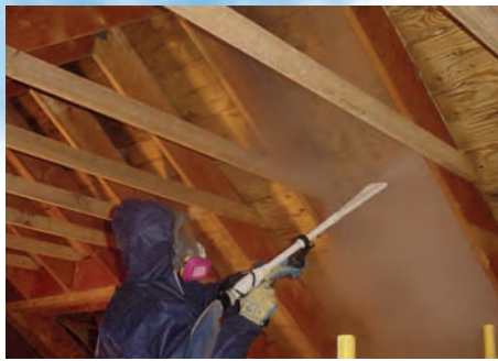
mold blasting - roof sheathing
