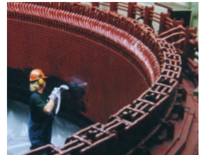
electrical - generator cleaning
